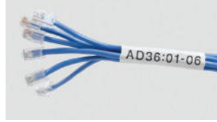
Heat shrink tube for cable identification
