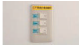
Power switch labels
